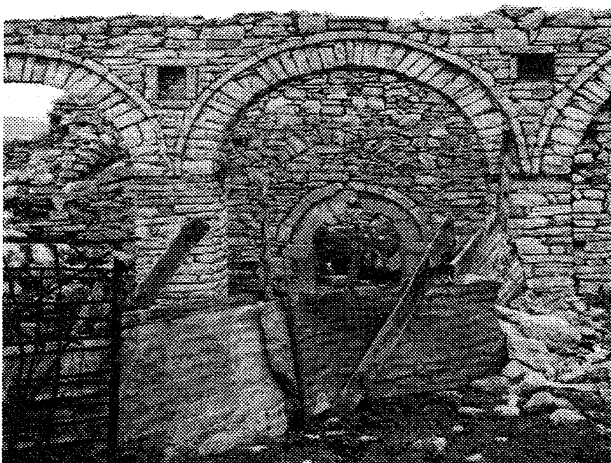
The ground floor of the meydan in the tekke of Dorbali Sultan
